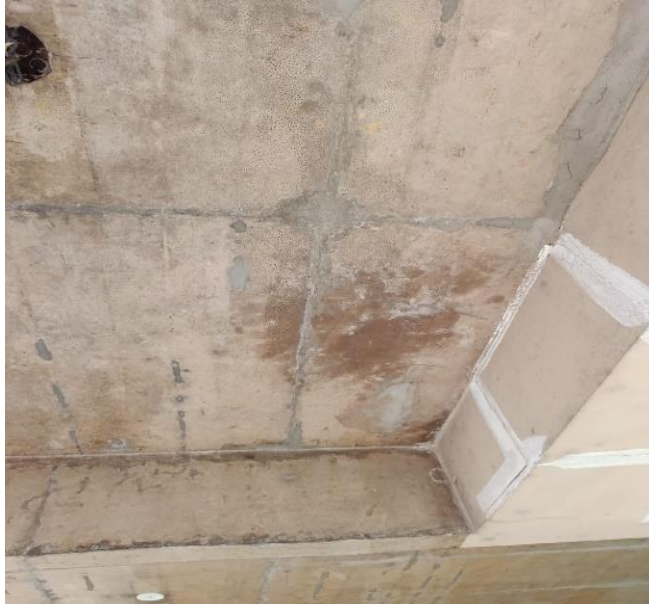
Figura 36 - Laje 1 - Manchas ( F_i = 2 )
